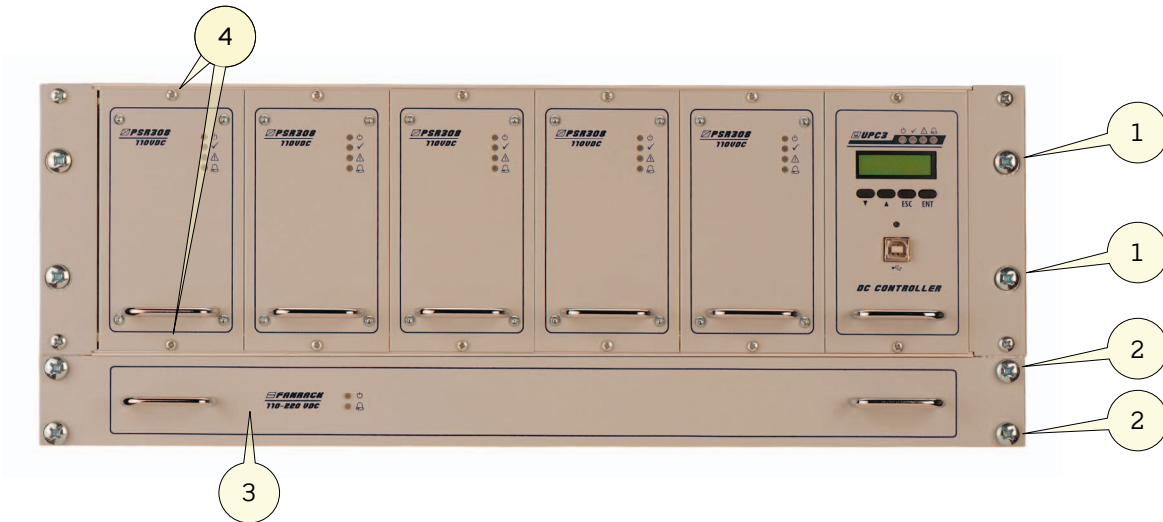
Figure 2) - DC power rack fully equipped with five rectifiers PSR308 and one DC controller UPC3S.
