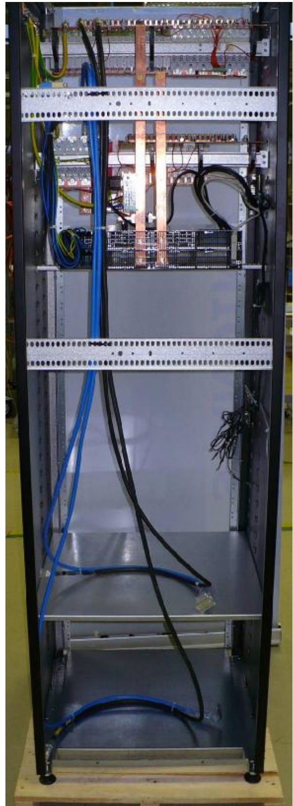
Back view without panels
